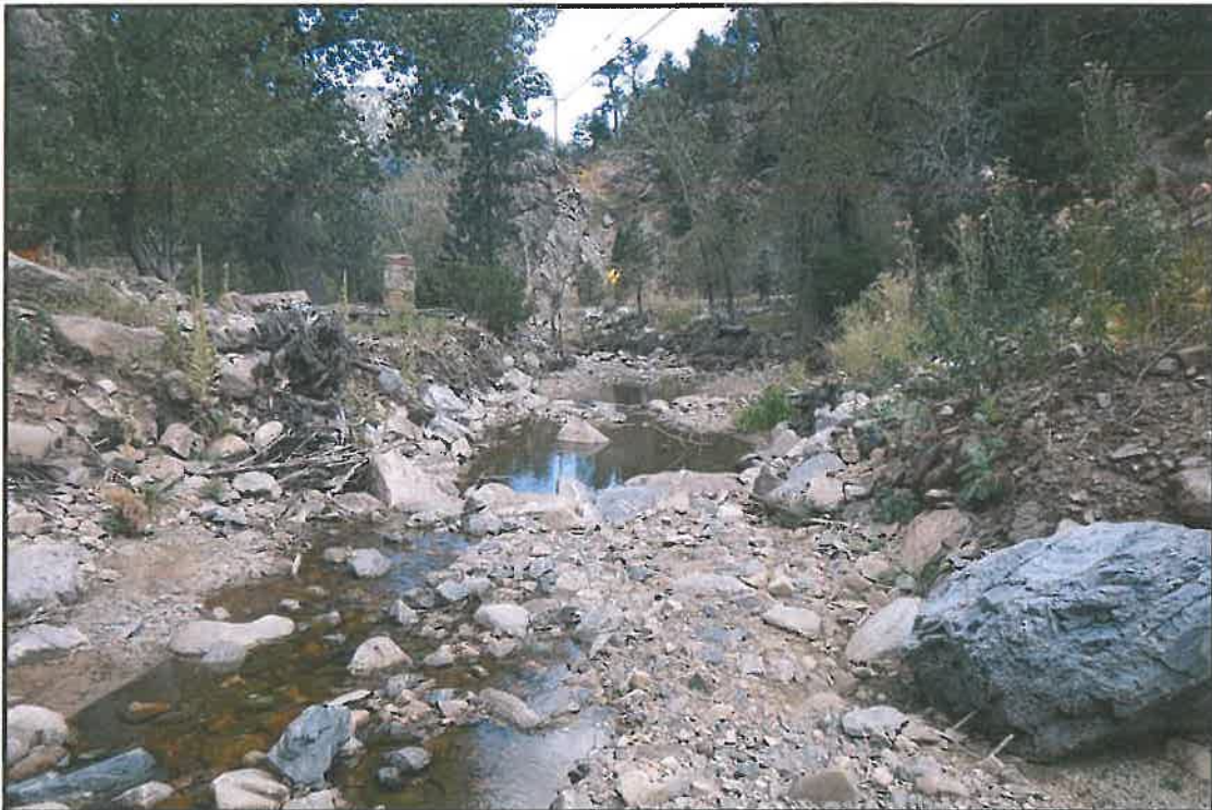
Overview of erosion and debris at the Start location.
