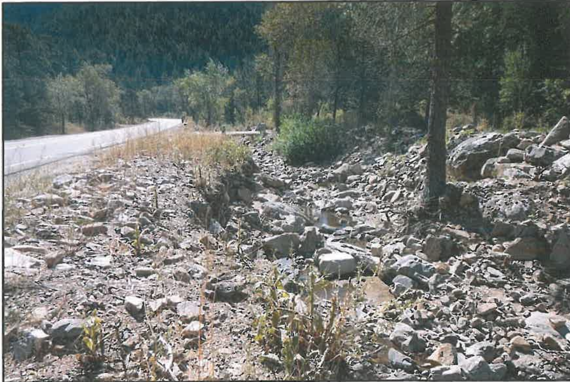
Closeup view of erosion adjacent to Highway 72.
