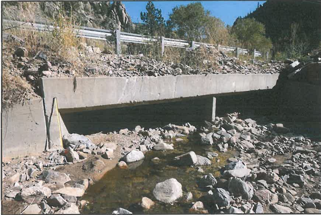
Closeup view of debris at road crossing at Start location.
