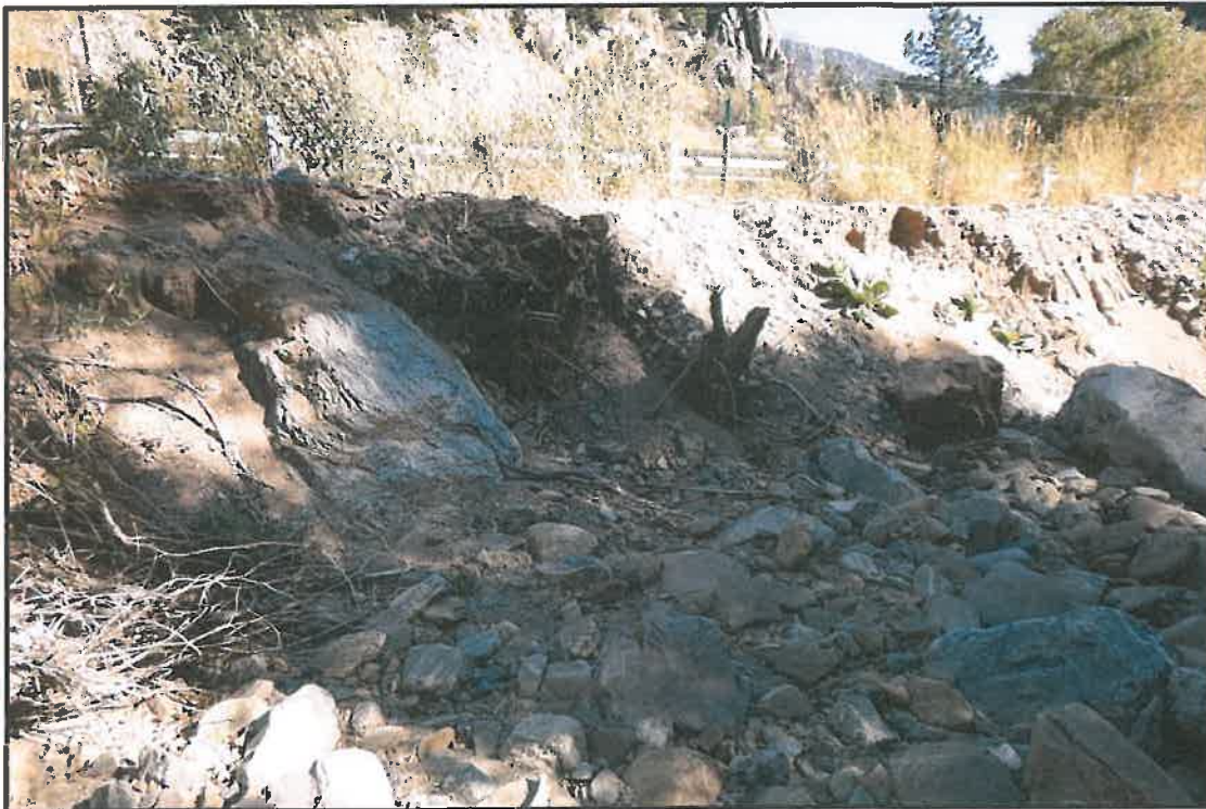
Overview of erosion along Coal Creek from 2013 flooding.
