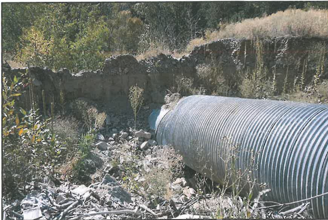
Closeup view of eroded and exposed culvert.
