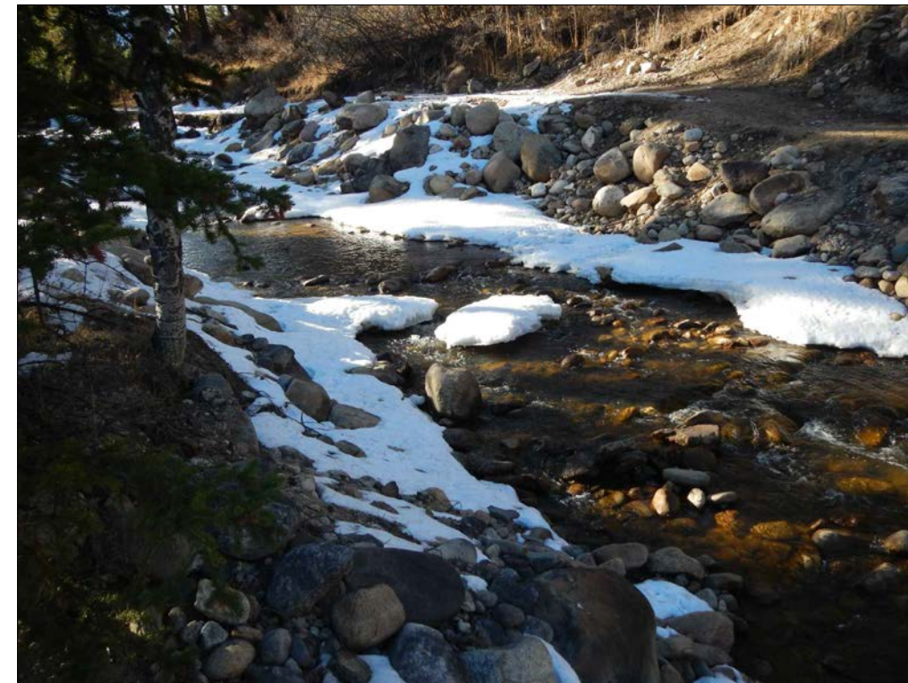
LARGE BOULDERS PLACED ON THE BANKS WILL BE REMOVED AND STOCKPILED FOR REUSE IN THE CHANNEL. RIPRAP WILL BE INSTALLED IN ITS PLACE.
