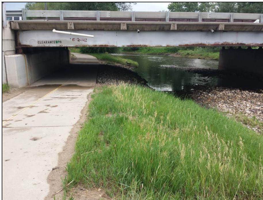
Figure 5.12. ACBs at bridge abutment, vegetated area in foreground covers ACBs.
