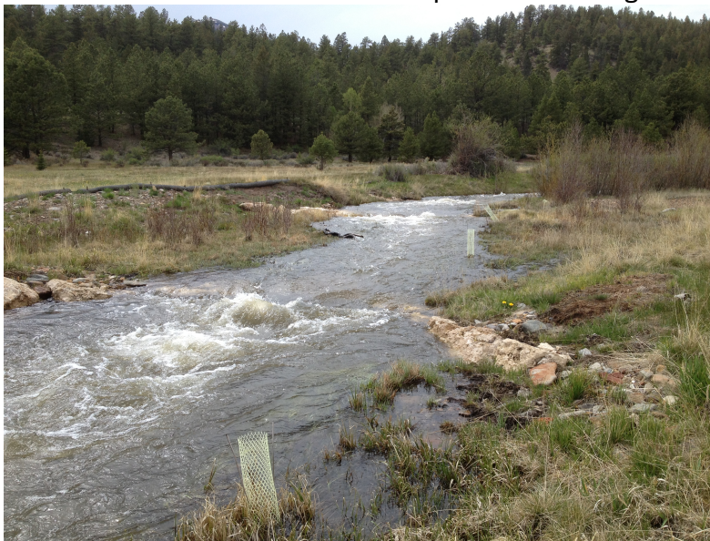
Picture 12: Example of streambank soil bioengineering on Kerber Creek in Villa Grove, Colorado
