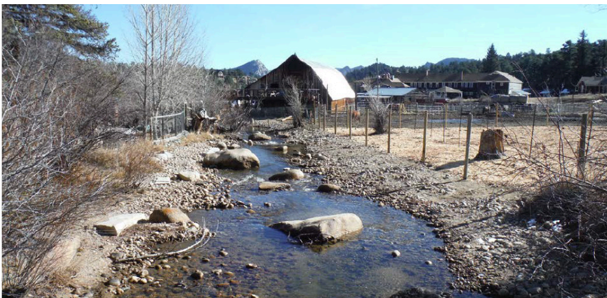
Below: Looking downstream from the Old Ranger Road Bridge after project construction (November 2017). Note the new fencing to exclude horses, removal of an old barn (left side of photo), boulder clusters, and riffle-pool sequencing.
