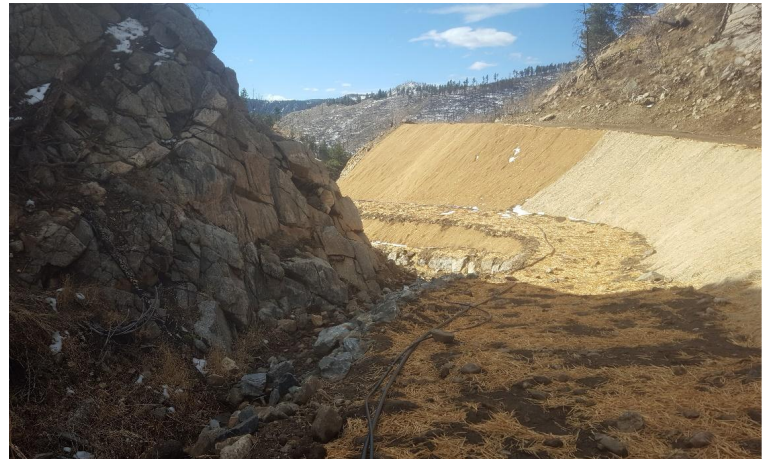
Stabilized section at the upstream end of the project reach showing grading of a landowner access route, steep erosion control blanket installation, and irrigation lines for watering.
