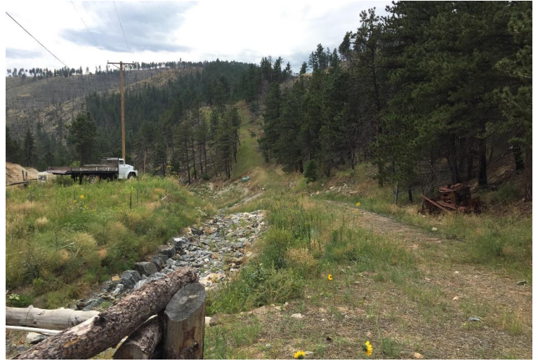
Lower portion of the project showing graded banks for flood conveyance, stabilized channel bed with in-stream grade control structures, banks protected with toe boulders and willows, and native revegetation throughout the reach.
