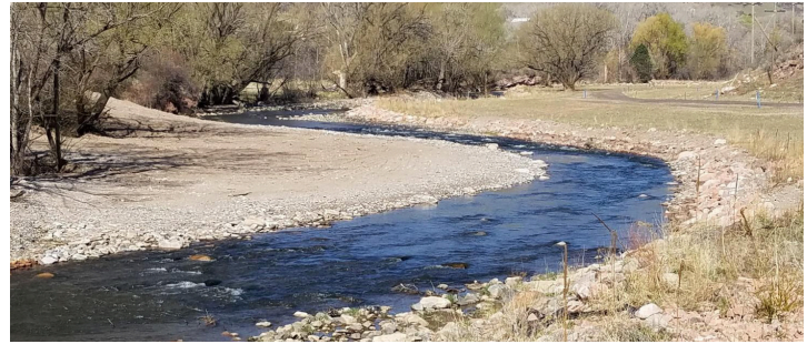
Channel realignment and point bar construction at City of Loveland water intake plant.
