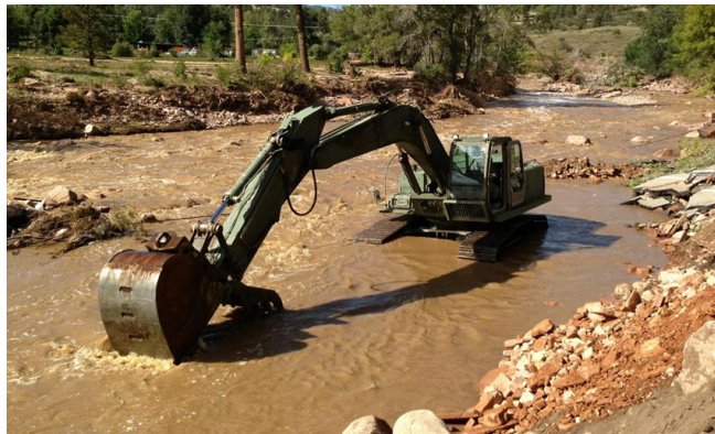
Above: Emergency repairs begin in Apple Valley very soon after the flood. Photo Credit: DARTW Public Affairs Office, 36th Infantry Division
