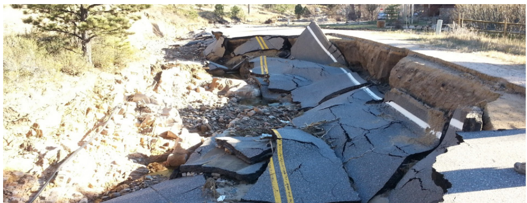
Destruction of Fish Creek Road as a result of the flood. Photo: Bill Spitz
