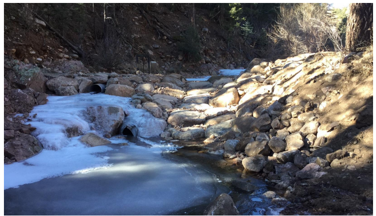
A new rock ramp has improved the long-term stability of the Gale diversion structure and provided the opportunity for improved aquatic organism passage.
