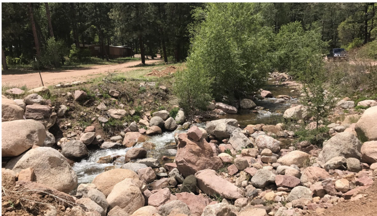
Looking upstream at channel in the vicinity of the May Museum parking lot.
