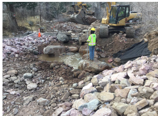
Left: A newly-constructed emergency spillway seeded and stabilized with erosion control fabric and hydromulch.
