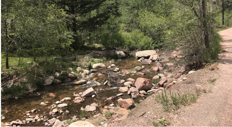
Looking upstream at a diversion structure that was flanked during the flood. Road repairs are temporary.
