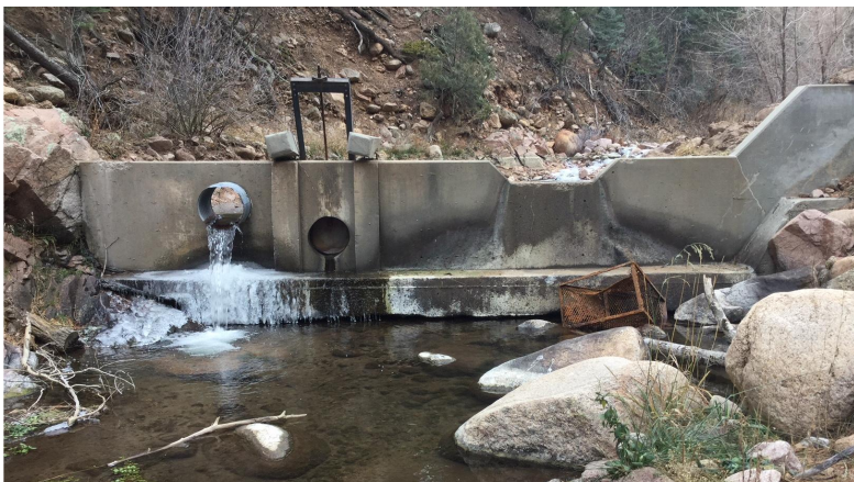
Excessive bed scour on the downstream side of the Gale diversion structure left it vulnerable to washout during the next flood.
