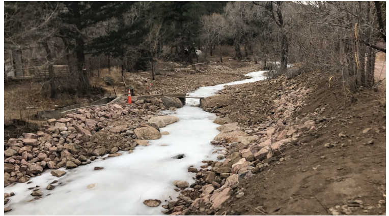
Looking upstream a repaired diversion structure and improved channel and floodplain capacity.
