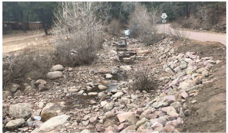
Looking upstream at reconstructed channel in the vicinity of the May Museum parking lot. Note improved channel capacity, grade control structures, and roadway embankment protection.
